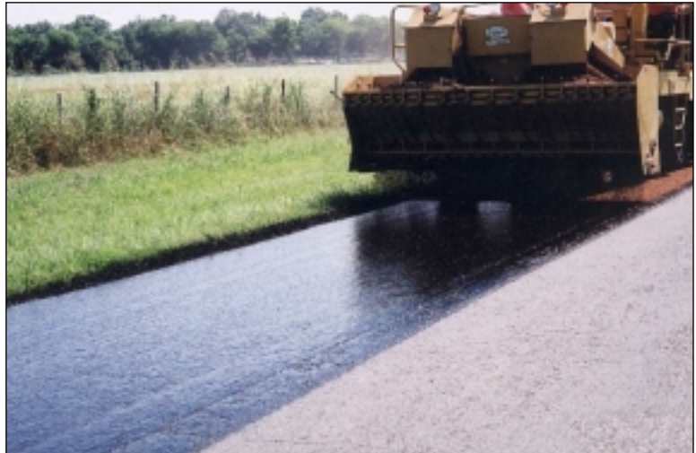
LITE-WATE being installed in Tulsa County, OK, near Memorial Street on 191 St. South. Emulsion placement rate @ 0.35 gal/sy
