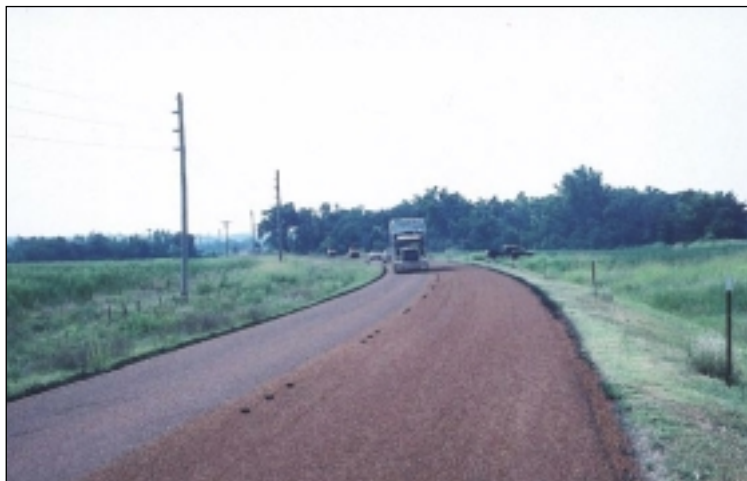
Traffic following a flag car on left. Road on right is 2 hours old, has been rolled, and will soon be broomed.
