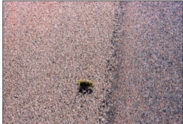
LITE-WATE aggregate on right is 4 days old. LITE-WATE aggregate on left is 1 hour old. Temporary center-line tab shown (lower center).
