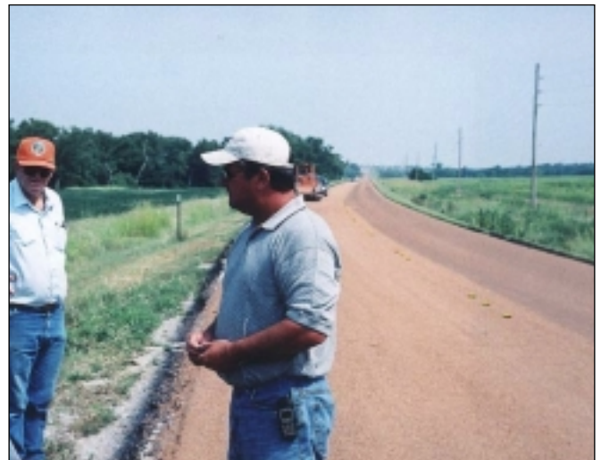
4-day-old placement on right shows emulsion has firmly "planted" the LITE-WATE aggregate. Chuck Loudermilk (foreground) is a visitor from ODOT, who is observing the Kansas-specified method of chip seal paving.
