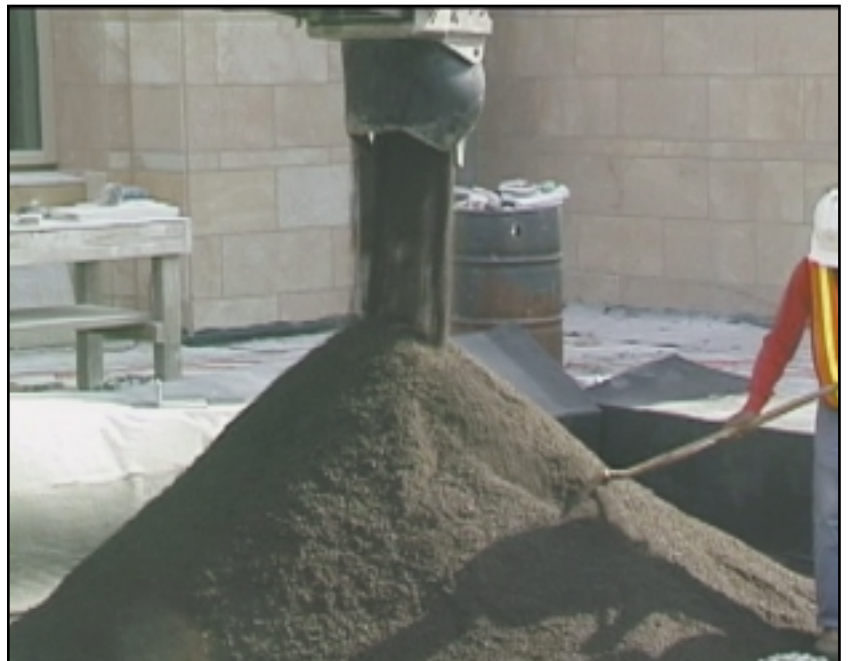
Lightweight growing medium is easy to place and compact, and provides a secure anchor for plantings
