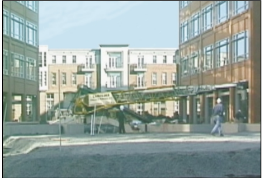
Putzmeister telescoping conveyor used to place lightweight soil mixture over underground parking structure
