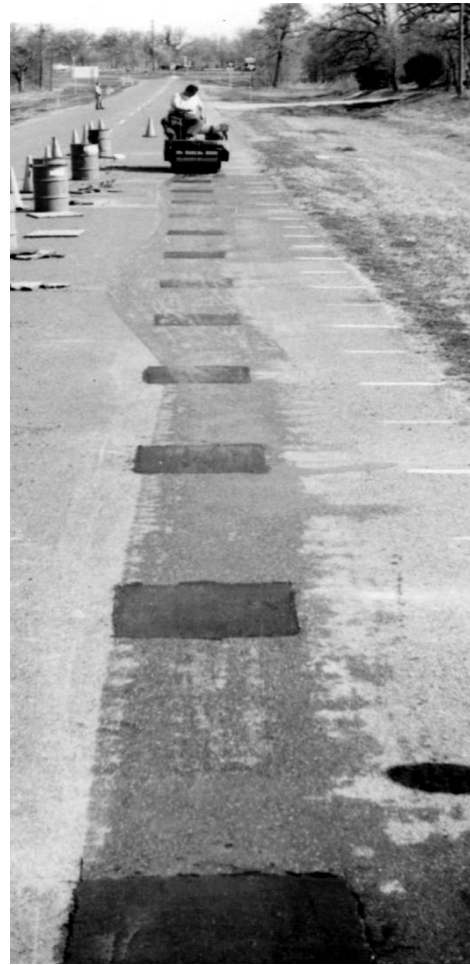
Figure 14.23 Completed patches where patching material had been in open storage for one year.
