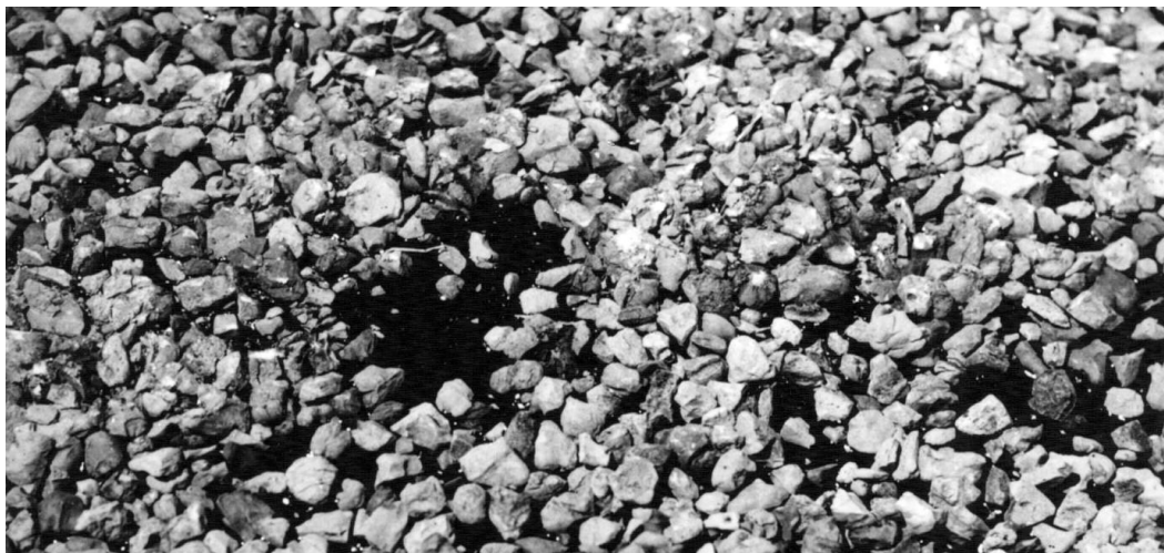
Figure 14.11 Road Surface before rolling showing what appears to be an inadequate aggregate cover
