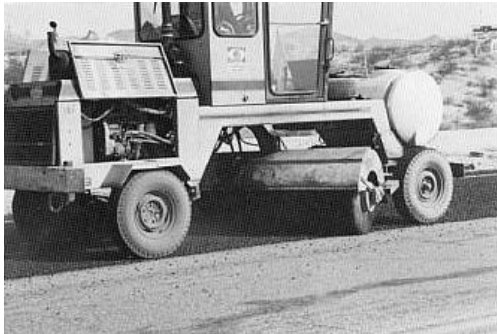
Figure 14.29 A self-propelled rotary "sidekick" sweeper broom removing loose aggregate from the pavement.
