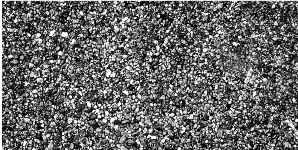
Figure 14.12 Same surface as Figure 14.11 after rolling and one month of light traffic
