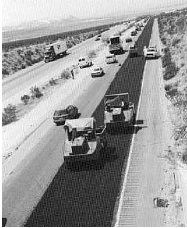
Figure 14.28 I-15 Asphalt-rubber chip seal project showing three pneumatic rubber-tired rollers following the chip spreader.
