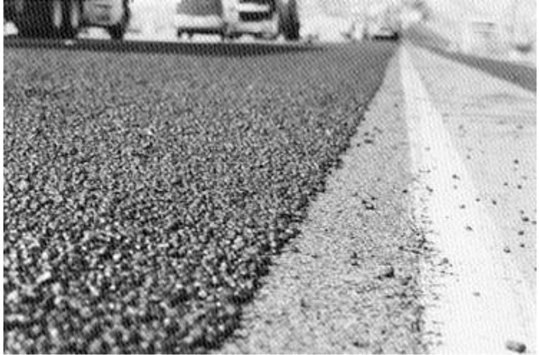
Figure 14.30 Longitudinal edge joint showing excellent adhesion, embedment and distribution of the aggregate in the asphalt-rubber binder.
