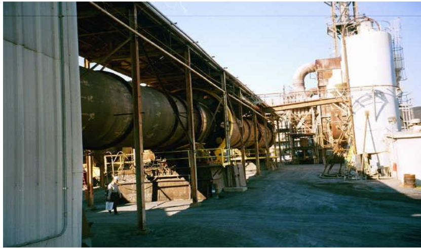
Figure 2.8. View of a Rotary Kiln Plant
