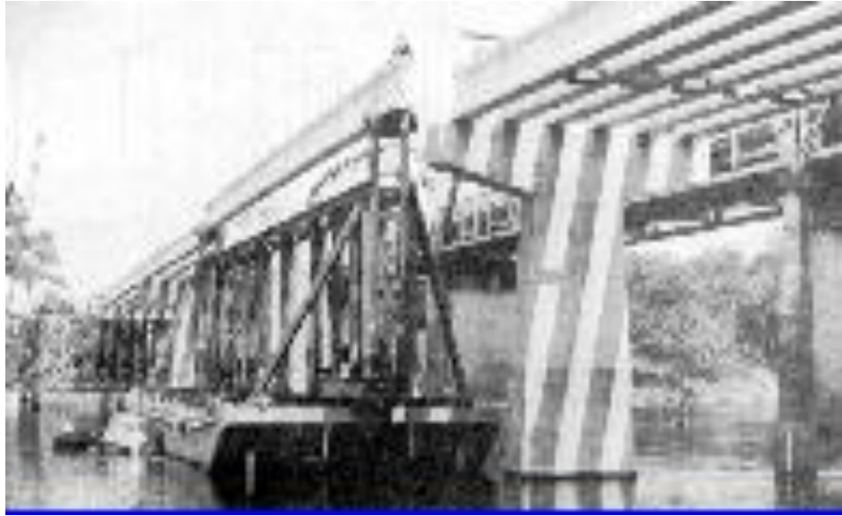
Figure 7.8. Barge-mounted frame placed lightweight concrete beams (to the right is an old truss bridge; both bridges will carry U.S. 19 traffic) (Brown, Larsen and Holm 1995)
