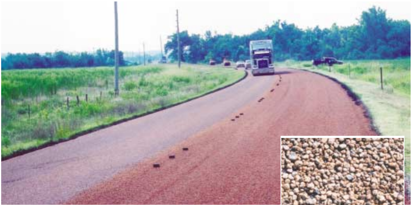
Traffic following a flag car on the left. Road on right has been rolled and broomed, is two-hours old, and about ready for traffic. (Inset) a close up one-hour old.
