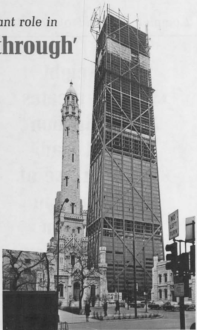
Contrasting vividly with Chicago's historic Water Tower, the John Hancock Center exhibits the bridge-type structure which will enable it to withstand high lateral forces against its 1,107-foot height. Lightweight concrete in floor slabs played important role in economy of structure, with unit costs comparable to those of buildings half its height.
