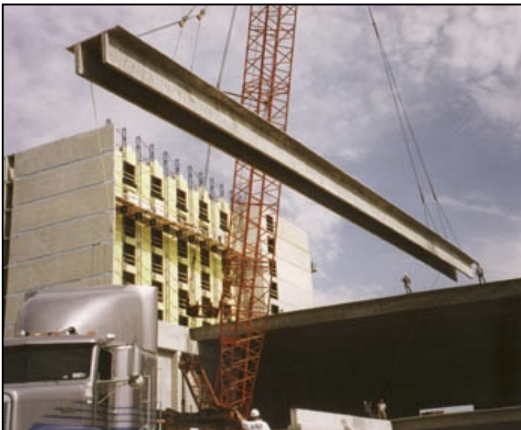
Installation of 8 x 4 ft (2.44 x 1.22 m) section, 128 ft. (39 m) long lightweight concrete double tee. (Photo: Jordan Phillips, Jordan Specialty Advertising)
