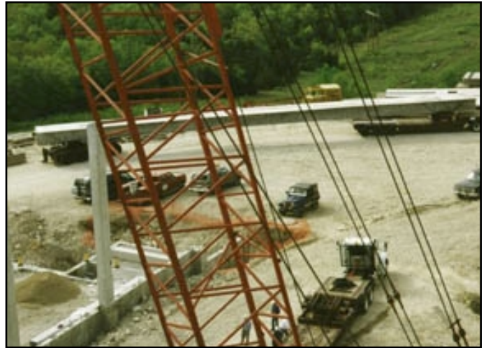
Arrival of lightweight double tee at site (Photo: Jordan Phillips, Jordan Specialty Advertising)
