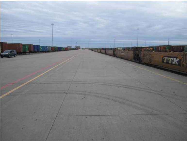
Figure 24. ICC pavement at the UP Intermodal Terminal showing rail cars on the right and truck containers parked on the left, with ICC pavement between them.
