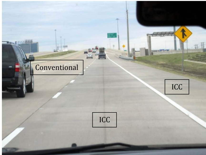
Figure 7. ICC placed in outer traffic lane and shoulder on Texas SH 121 in 2006.
