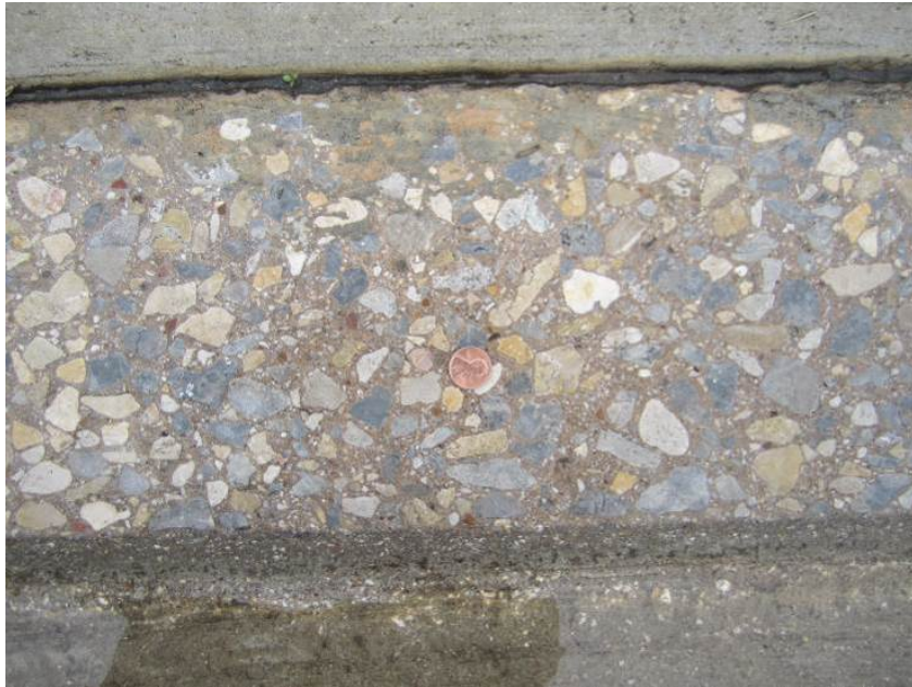
Figure 36. Ground-off conventional concrete without LWA at Alexandria Meadows.
