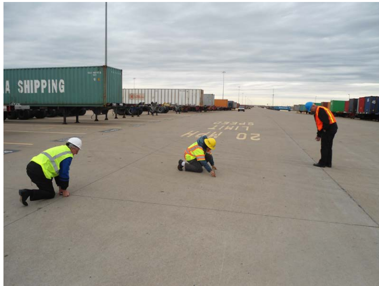
Figure 26. Measuring diagonal corner slab upward curl at the UP Intermodal Facility. No upward curling was measured on 20 slabs around the facility.
