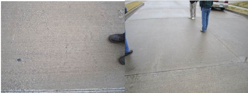
Figure 37. Small shrinkage cracks found on Alexandria Meadows on ICC pavement (Left) and conventional concrete pavement (Right).
