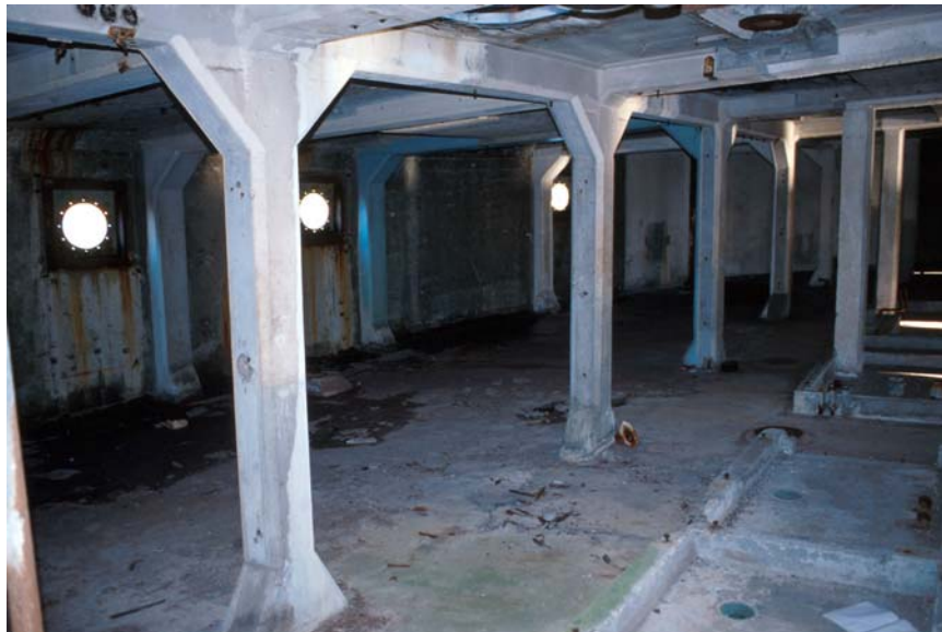
Fig. 6 View of the interior of a cabin on the Emile Vidal shows minimal deterioration of surfaces protected from rain and seawater.
