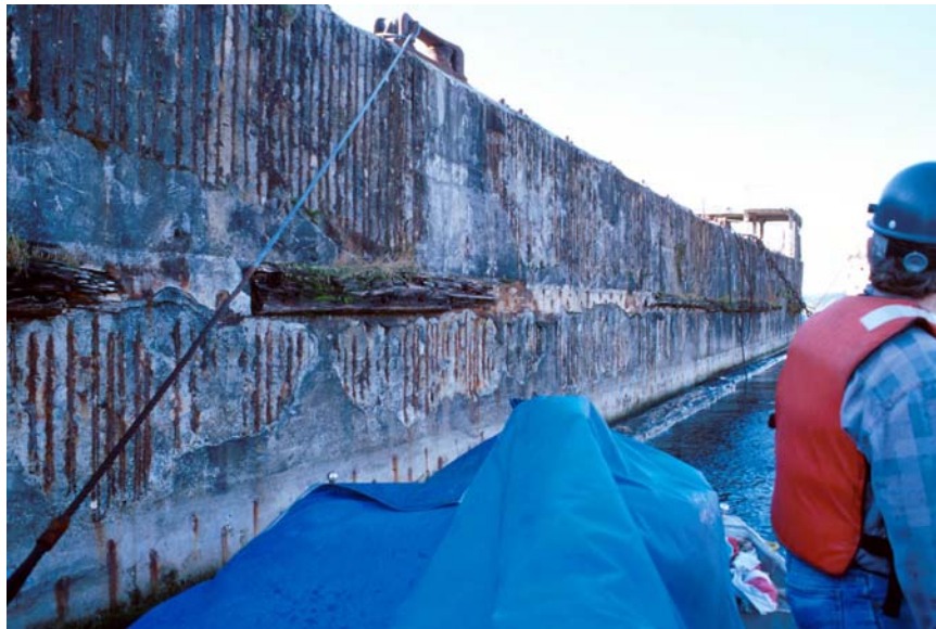
Fig. 3 Severe spalling along the hull of the Emile Vidal exposes corroded steel reinforcement. Most of the surface distress on the other ships built in the 1940's is not so severe.
