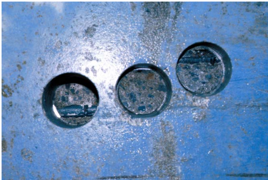
Fig. 4 Photograph shows steel reinforcing bars exposed by coring along the hull of the Yogn are in good condition with negligible corrosion.
