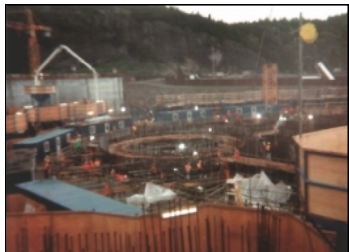
Tight schedule maintained by intensive round-the-clock construction of the GBS in “dry dock”
