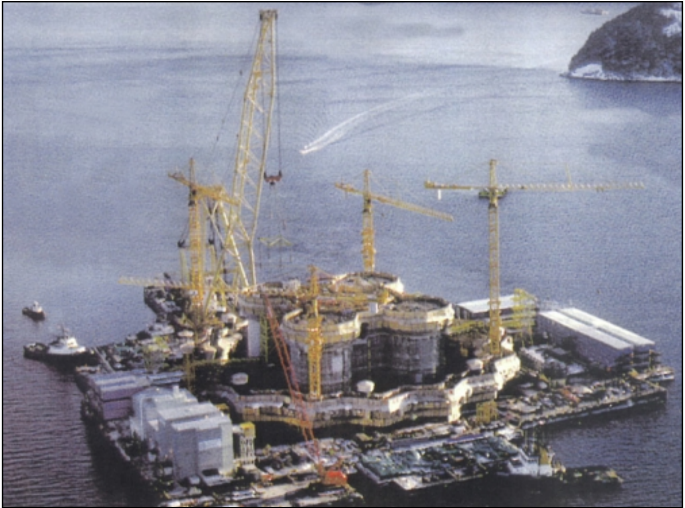
The GBS was floated and towed into a deep water harbor for construction completion.
