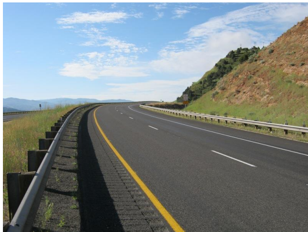
I-80 near Coalville, Utah exactly 1 year after being chip sealed with ESCS lightweight aggregate in 2010. Picture taken in August 2011.
