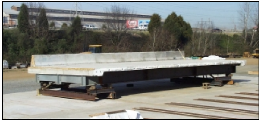
Precast structural lightweight concrete span section with attached steel bridge supports as seen in casting yard
