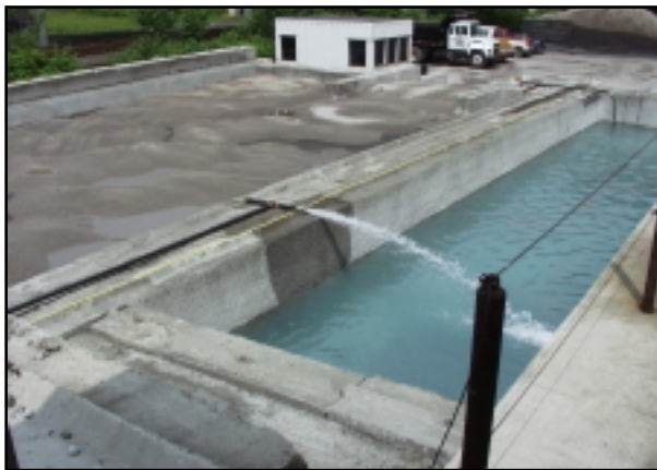
Pumping water out of saturation pond to prepare Lelite lightweight aggregate for lightweight concrete placement later the same night.
