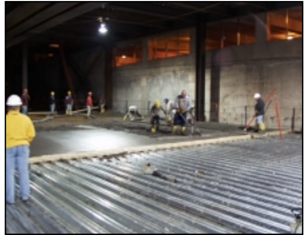
Shelley Sheetz, Lehigh representative, observing lightweight concrete placement for new second floor of Hilton Hotel ballroom
