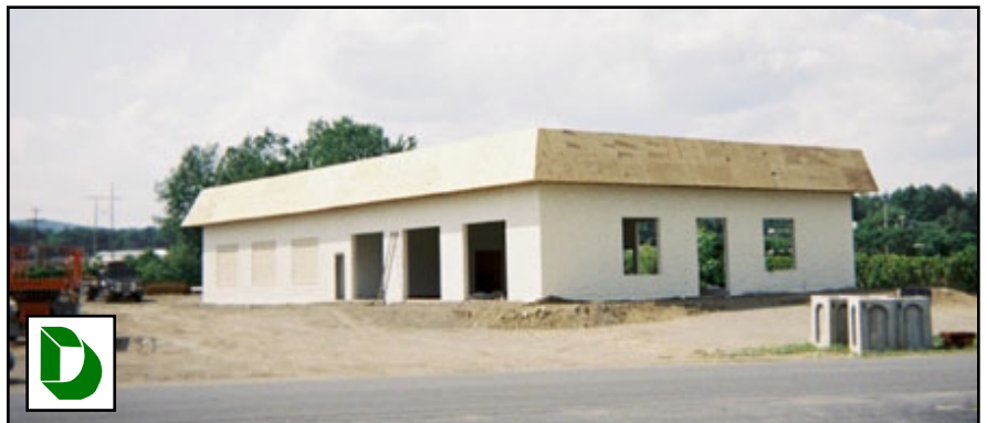
Second Warren Tire Service Center (under construction), Queensbury, NY, 5,000 ea. 8" SmartWall Splitface block with paint.
