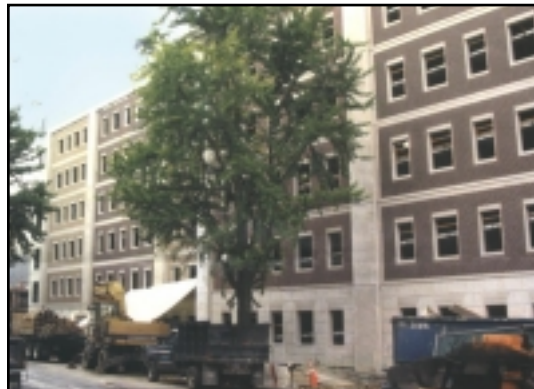
Parking garage as seen from Martine Ave. Exterior thin brick spandrels are shown.
