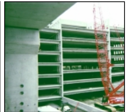
1,100 lightweight double tee deck members were used to reduce dead load and improve fire rating.
