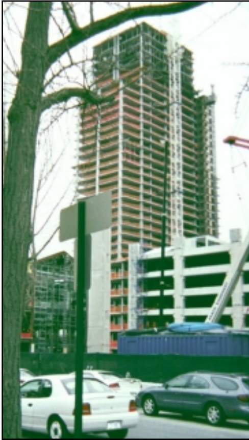
One of City Center's two 35-story towers rises behind the structural lightweight concrete parking structure
